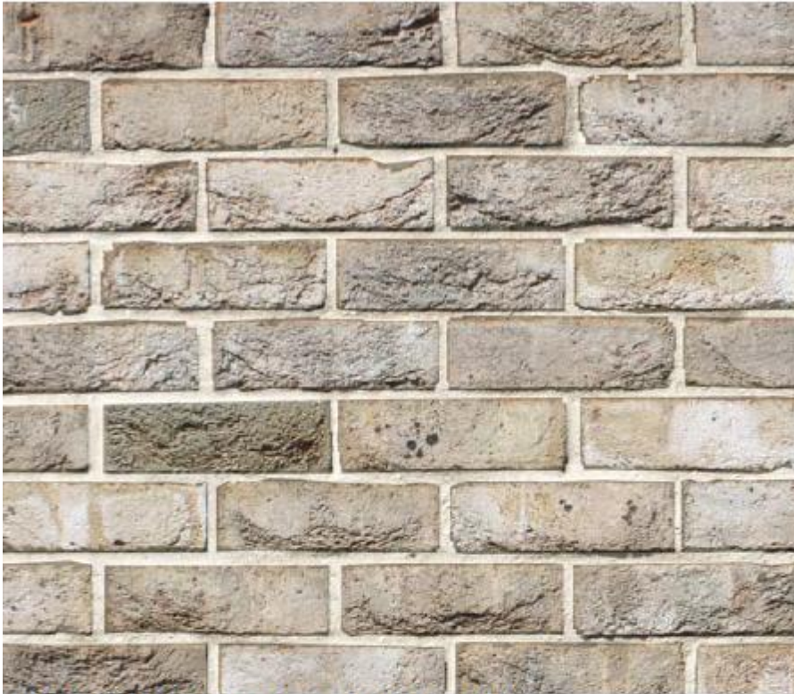
Buff brick with a lighter natural mortar used on the taller buildings
